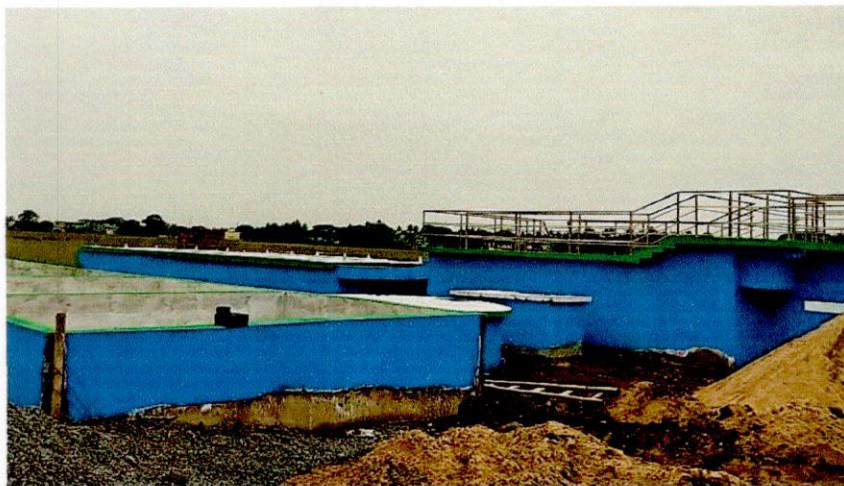
Fig.-7- A view of the newly constructed FSTP by Kendrapara Municipality
