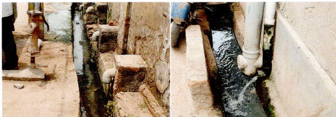
Views of domestic wastewater drains connected with the municipal drain at Naya Idgah
