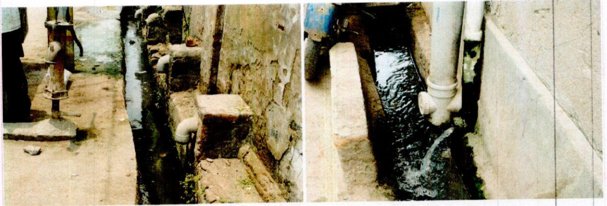
Views of domestic wastewater drains connected with the municipal drain at Naya Idgah
