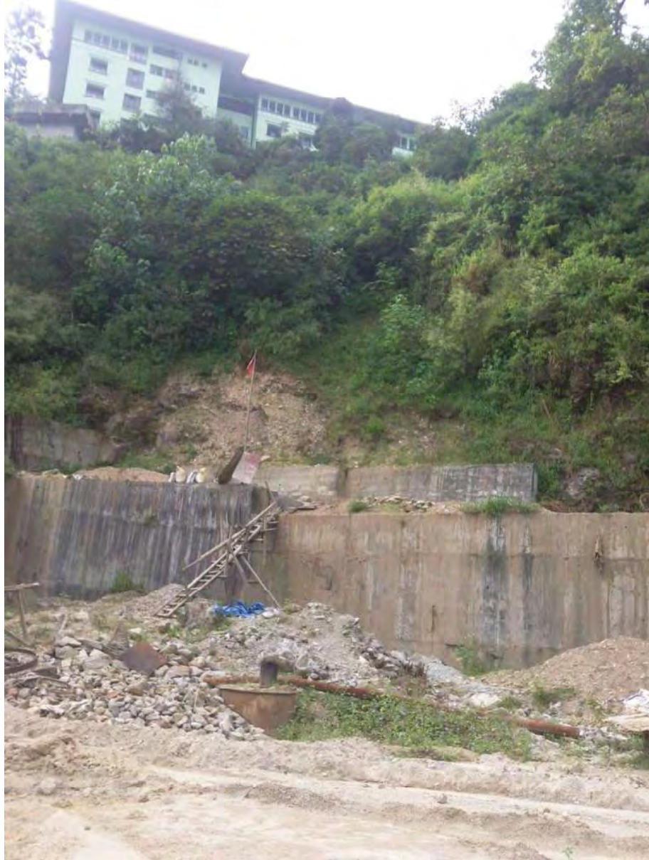
Fracture plane (Wedge Failure in In-situ rock formation) towards South West of Present Secretariat.
