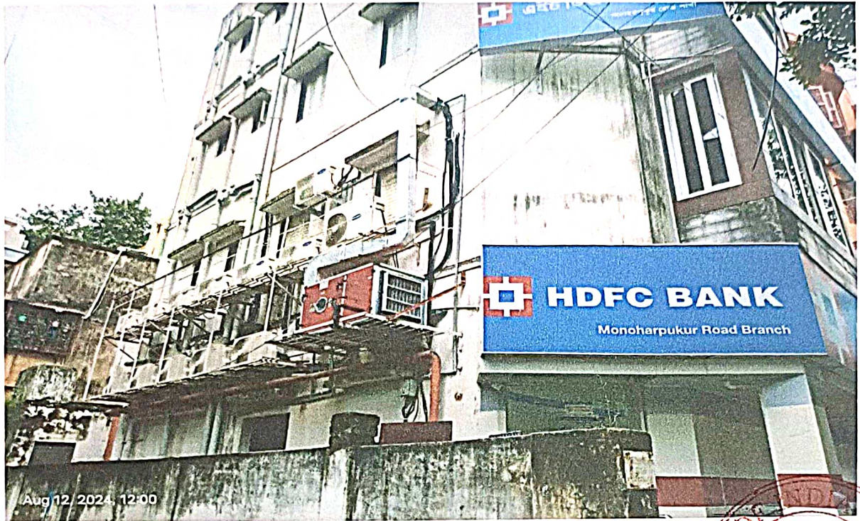
Outdoor units of A/C machines on the western wall of HDFC Bank.
