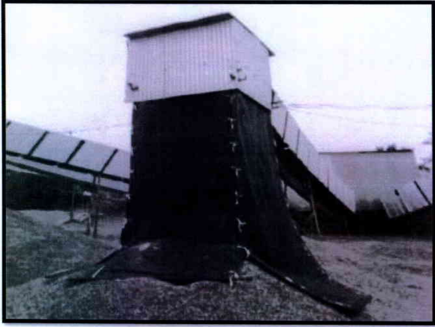
Figure-2: Chute from top of discharge point
