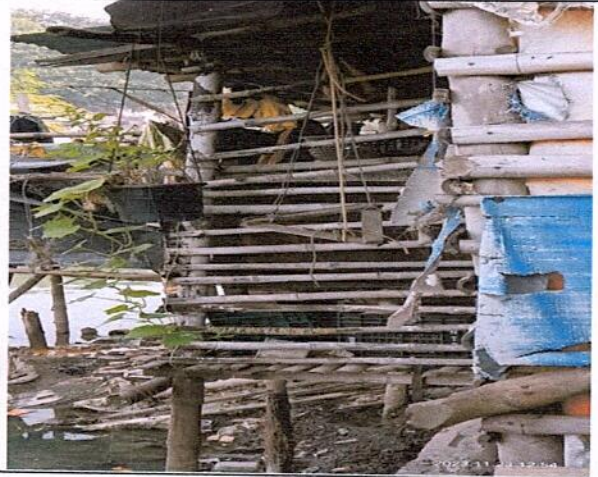
Close up of encroachment of bank of canal
