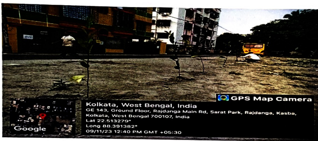
Photograph after removal of silt/slush, spreading of silver sand and starting of plantation.
