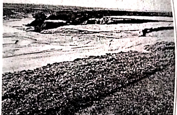
No free board at this location of Ash Pond-C
