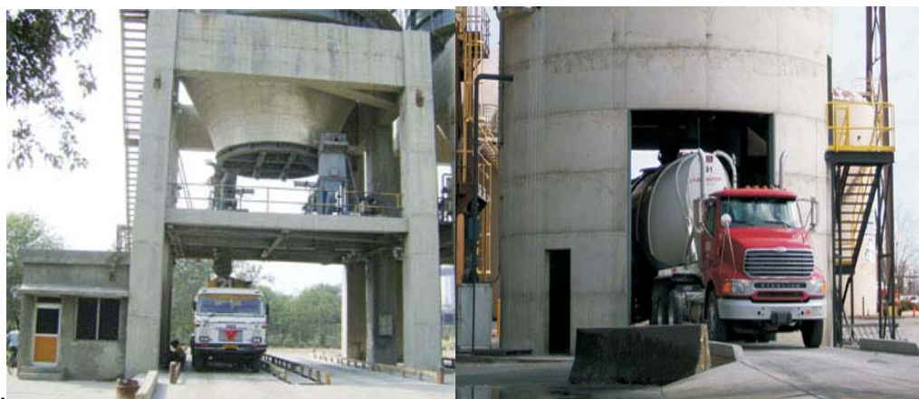
Photograph showing flyash loading into truck & bulker through telescopic chute avoiding fugitive emission
