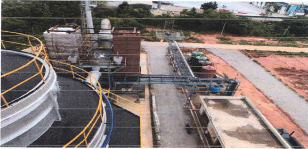
Photo 7: H.W. Incinerator overview showing Bag house, chimney, caustic storage tank etc.
