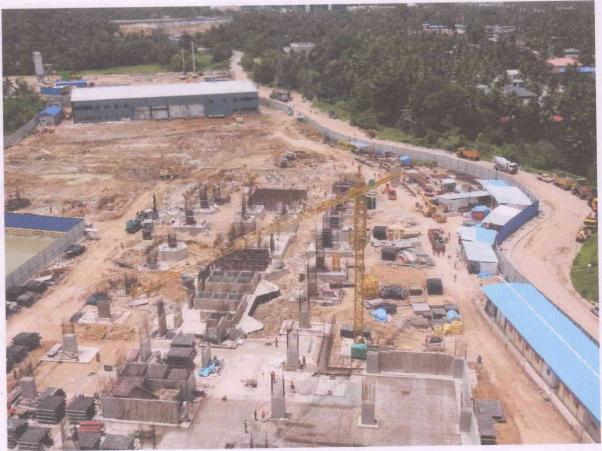
Construction activities in the Special Economic Zone (SEZ), Phase III expansion of Technopark, Trivandrum
