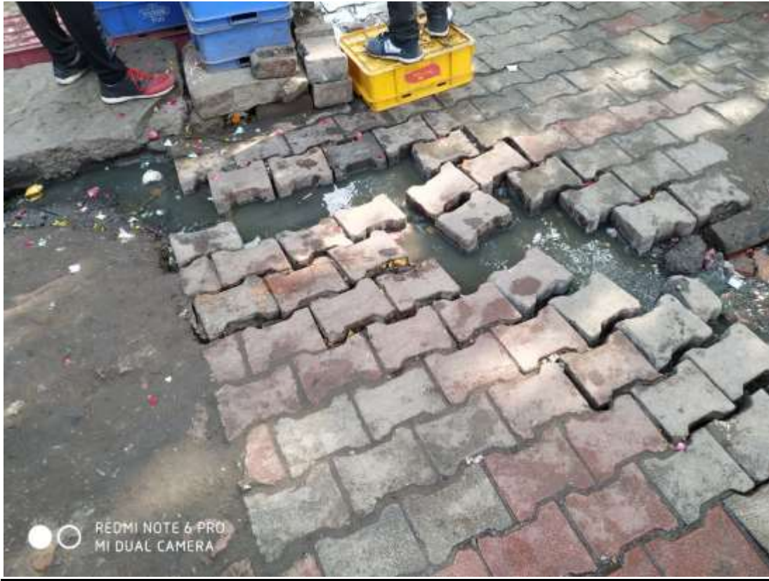
NEWLY CONSTRUCTED PAVMENT : WATER FLOWING IS FROM SEWAGE
